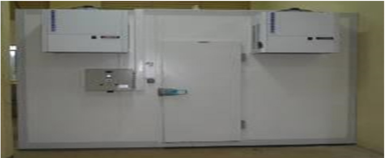
Figure 6-2 Cold room/freezer room
