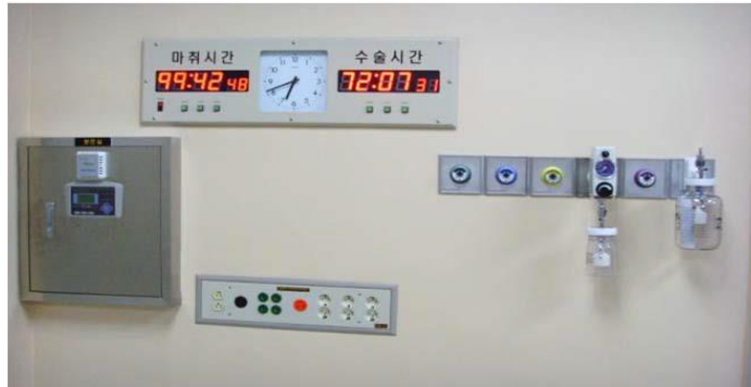
Figure 4.10: Pipeline inlets, pipelines, 50psi and pressure gauges
