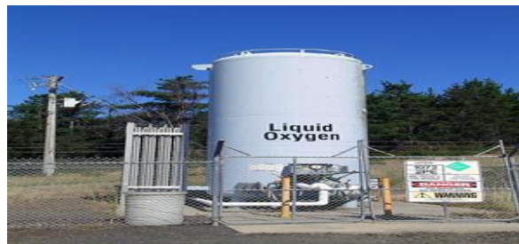
Figure 4.9: Central gas supply for oxygen
