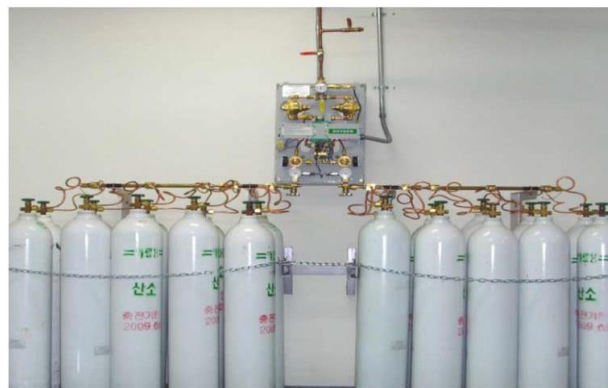
Figure 4.7: Medical Gas Supply Facility Room
